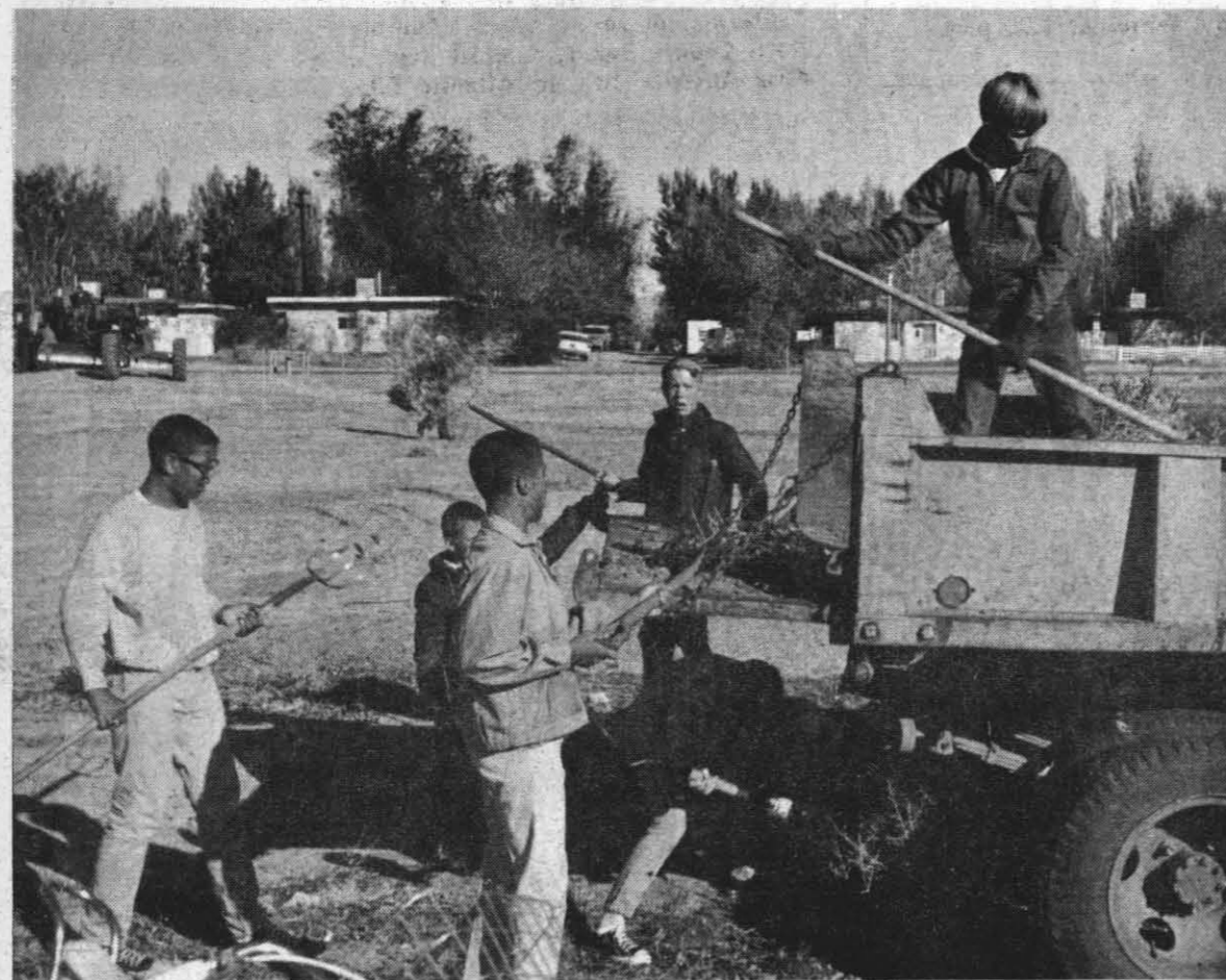
BOYS BUILD A BALLPARK — Assembling a petition signed by more than 300 parents, boys of Capehart "B" area asked the Community Council to help them obtain a playground. With assistance from the Public Works Engineering Division, Maintenance Control Division and the local Naval Reserve Seabee Unit 11-2, the boys cleared
