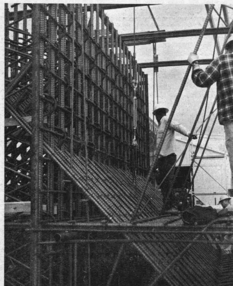
HAND-TIED STEEL — The maze of hand-tied steel reinforcing bar dwarfs Public Works riggers as they prepare 44-foot long structure for delivery to Systems Development Department at Naval Weapons Center.
