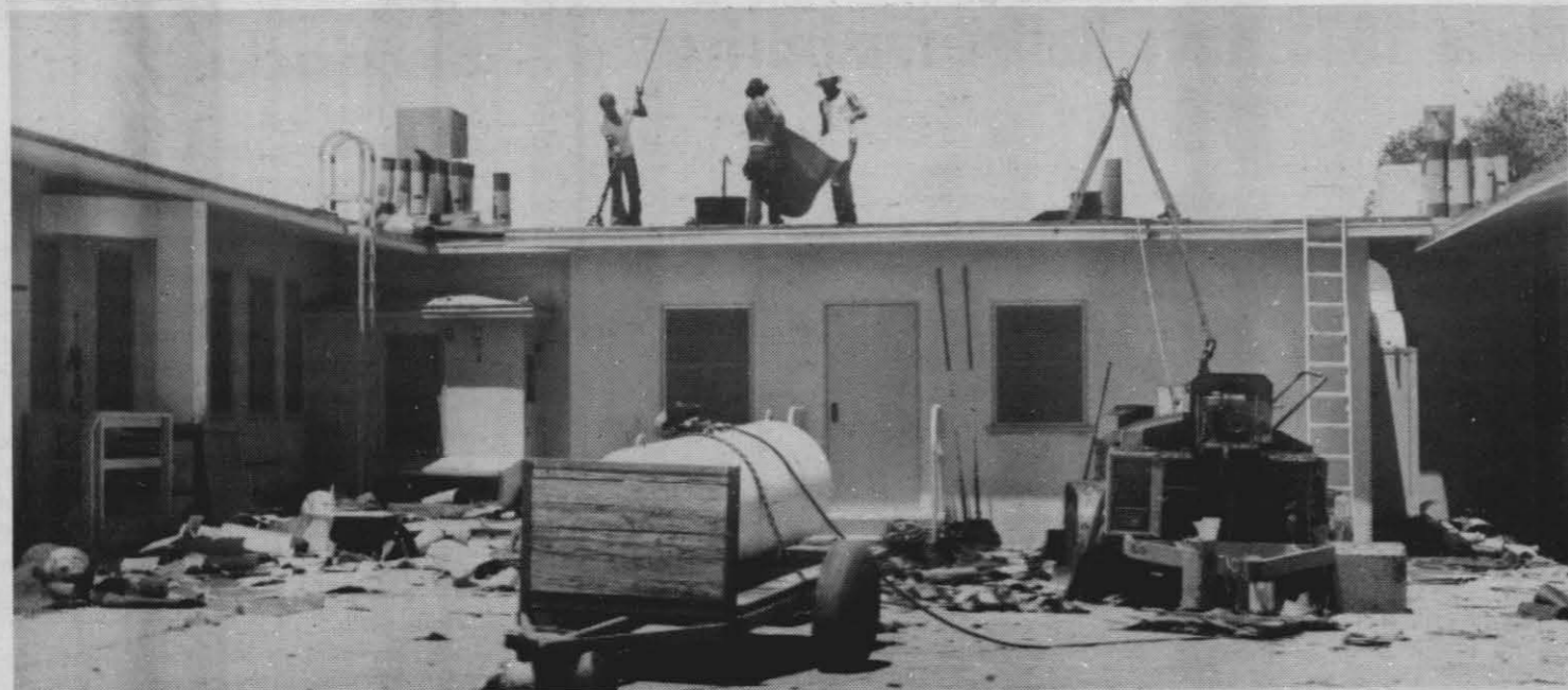
REMODELING JOB — Workers tar the roof on the old NWC Dispensary building, which is being refurbished to accommodate employees of the Technical Information Department. Remodeling of three of the building's wings is scheduled for completion in late August. The first group of 60 TID employees is slated to move in during September.
