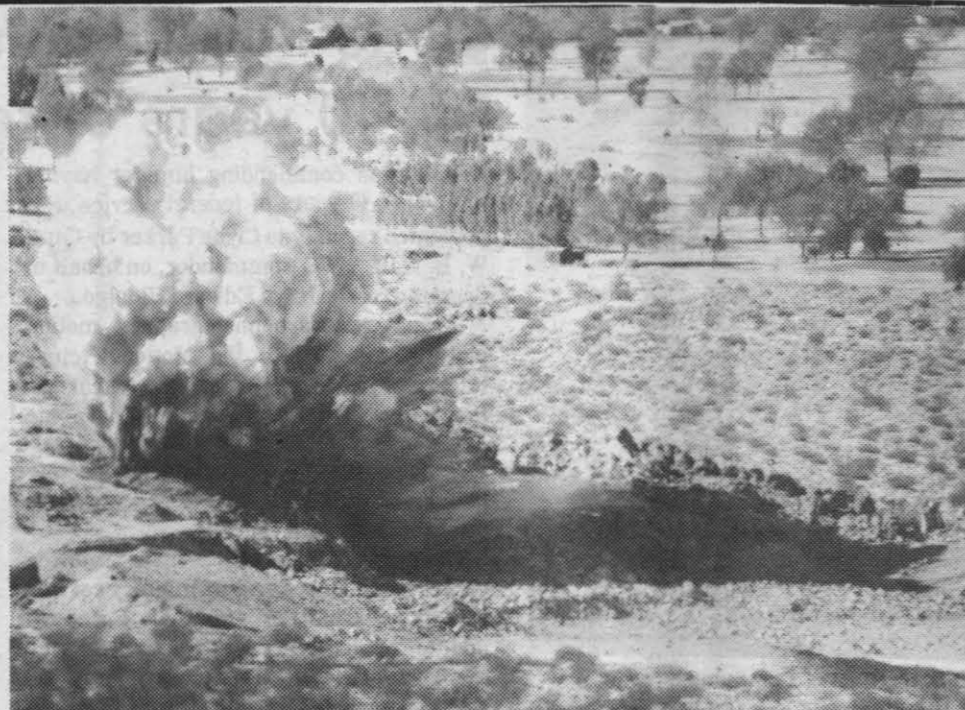
THERE SHE BLOWS — In preparation for the work of installing an asphalt concrete overlay on runway 3-21 at Armitage Airfield, the contractor (Desert Construction of Victorville) is blasting rock from a quarry site located east and north of the China Lake golf course. The rock from the quarry must be crushed and screened before mixing it with asphalt to form a part of the 2-in. thick overlay. The job calls for preparation of the existing runway surface to accept the overlay, as well as some leveling work where the airfield runways intersect. It may be mid-January before the actual work on the airfield runway begins.
