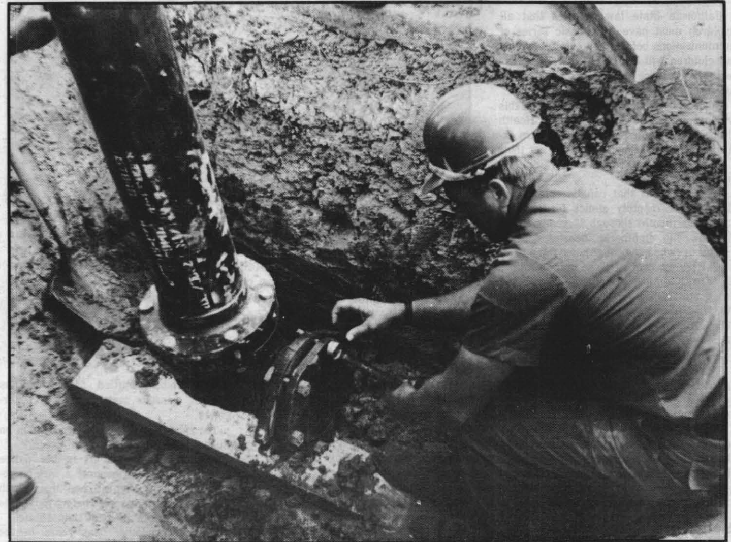
NEW HYDRANT — UT3 Dave Stallin prepares the slip coupling prior to installation of a new fire hydrant at the U.S. Naval Station, Panama Canal. — Photos by CM1 Jerry Morrison, BU3N L. D. Yates
