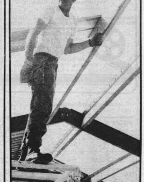
ON TOP — CE2 Marvin Windsor found himself at the top of things while working on the roof of the Butler Building.
