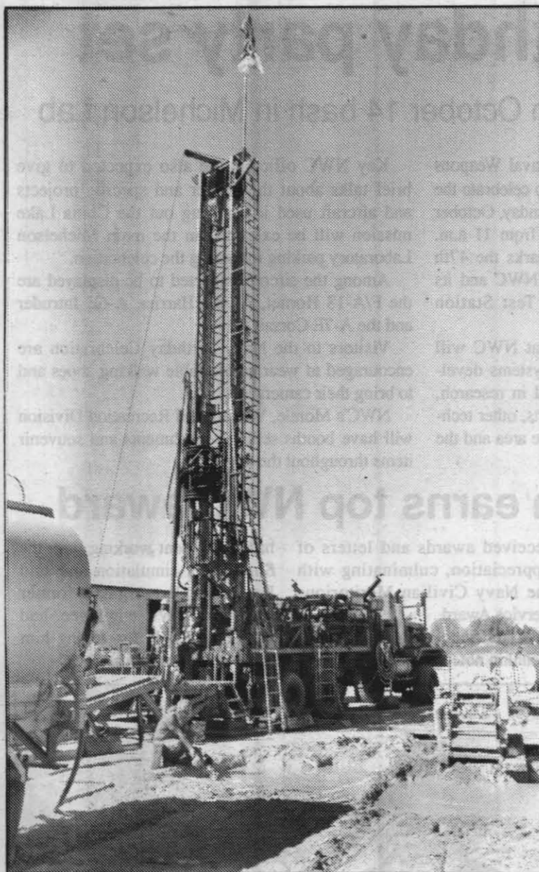
MONITORING WELL --Drilling crews hired by the Bureau of Reclamation began work on the first of as many as 10 monitoring in the IWV. NWC, Kerr-McGee, IWV Water District and the bureau share the costs. Photo by PH3 Cary Brady
